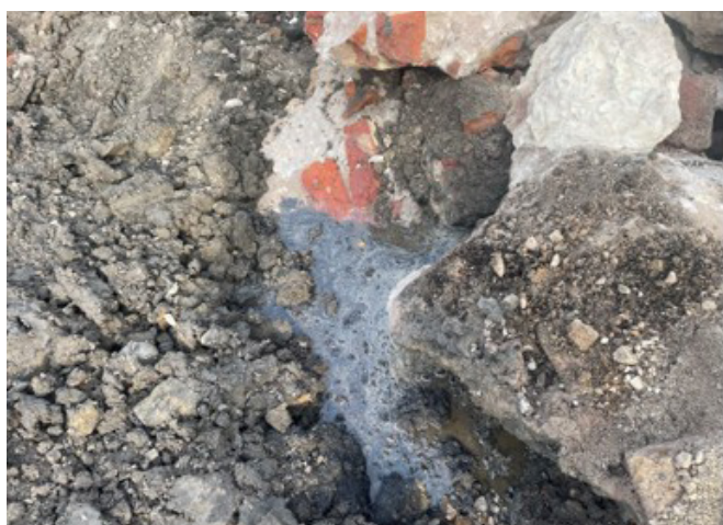
UNEXPECTED UNDERGROUND STRUCTURE AND CONTAMINATION
