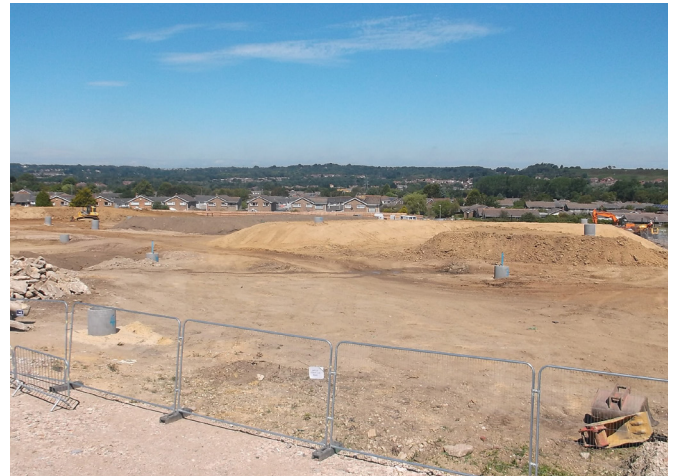
INSTALLED SETTLEMENT MONITORING POINTS
