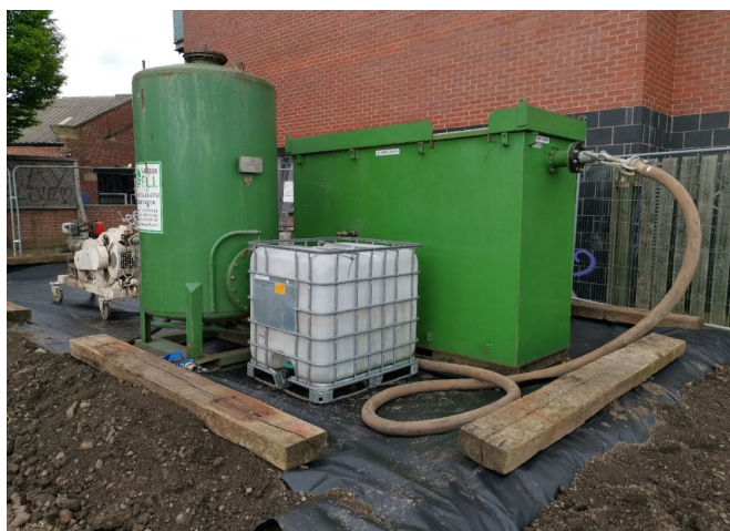
WATER TREATMENT PLANT COMPRISING OIL / WATER SEPARATOR, GRANULAR ACTIVATED CARBON POD, PERISTALTIC PUMP, FLOW METER AND STORAGE CONTAINERS
