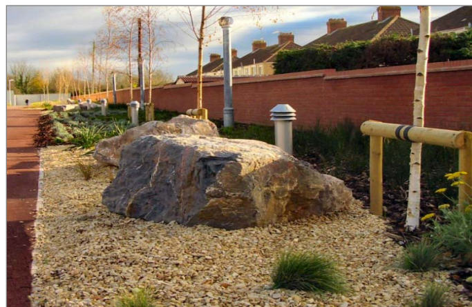
COMPLETED VENT STACKS AND VENT BOLLARDS IN LANDSCAPED AREAS AROUND ASDA SITE
