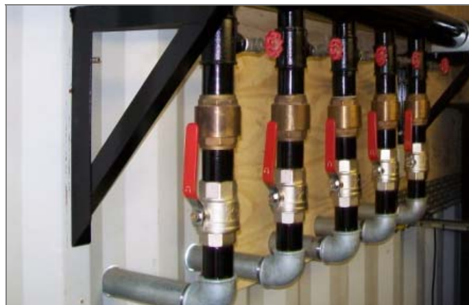
SOIL VAPOUR EXTRACTION MANIFOLDS
