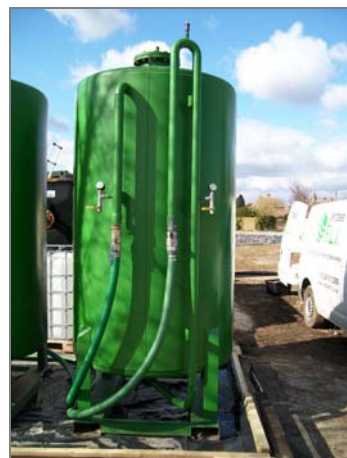
GROUNDWATER TREATMENT CARBON POD
