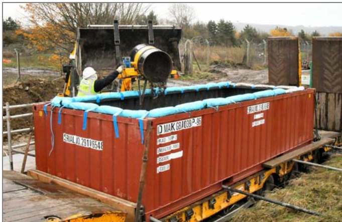
DECANTING LLW FROM DRUMS TO HHISO
