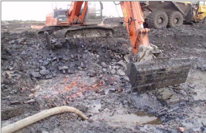
EXCAVATION AND SEGREGATION AT SOURCE OF IMPACTED SOILS AT BASE OF MADE GROUND
