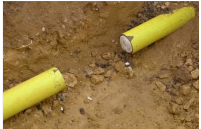
BURIED PIPE – SEVERED AND SHOWING FOAM FILL
