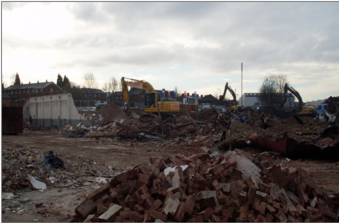
DEMOLITION OF FACTORY UNIT AND STOCKPILING OF MATERIALS FOR CRUSHING AND RECYCLING
