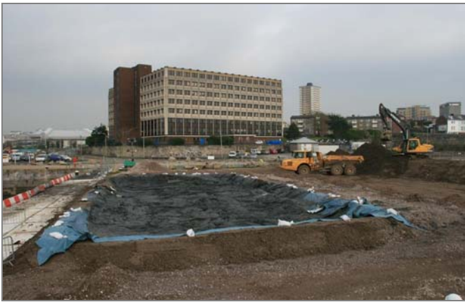
TEMPORARY STORAGE LAGOON FOR DREDGINGS PRIOR TO TRANSPORT TO PERMANENT STORAGE LAGOON
