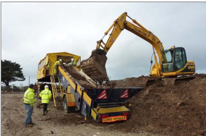
LOADING PICKING STATION
